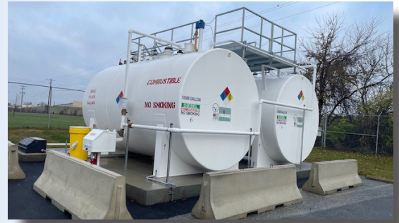
The two new diesel tanks installed at the RRTA Operations Center, 45 Erick Road, Lancaster.
