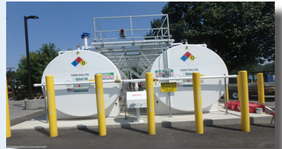
The two new diesel tanks installed at the 1700 N. 11th Street Reading facility.
